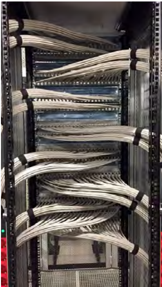
Proper rack cable management
