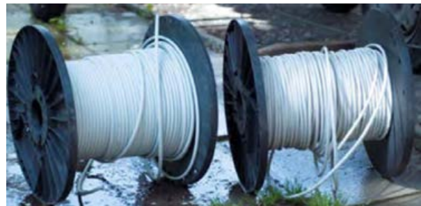
Copper cable stored in the wrong conditions
